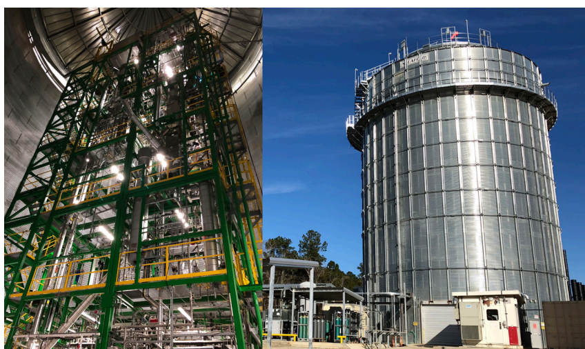
Figure 3. T-Cat-8 pilot plant.
